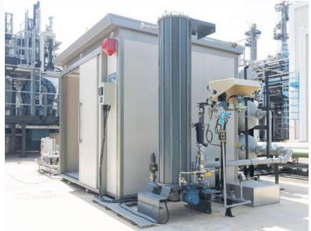
大埔煤氣廠內設置的煤氣管網取氫系統 Hydrogen extraction system from gas network located in Tai Po Gas Production Plant
